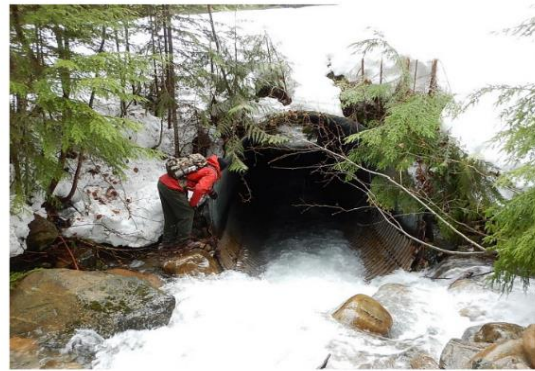
Undersized culvert inlet pre-replacement.
